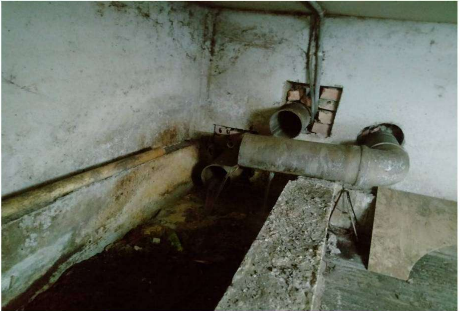
Internal sewer and storm water line
